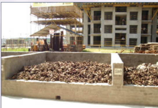
Material recovery tank
