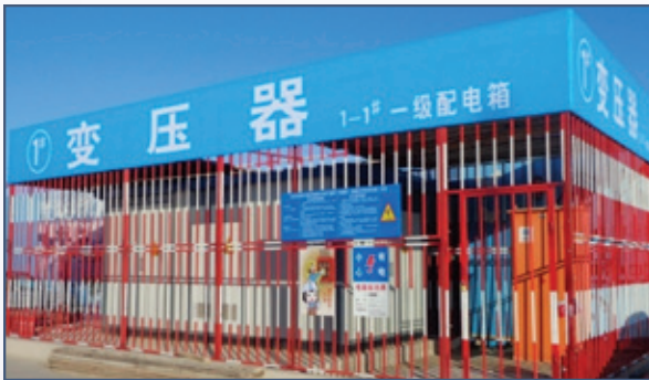
Protection for box transformer
