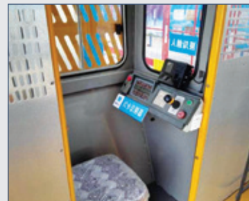
Driver of construction elevator face recognition system
