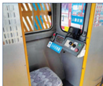
Driver of construction elevator face recognition system
