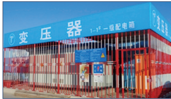
Protection for box transformer
