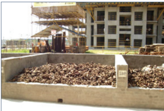
Material recovery tank
